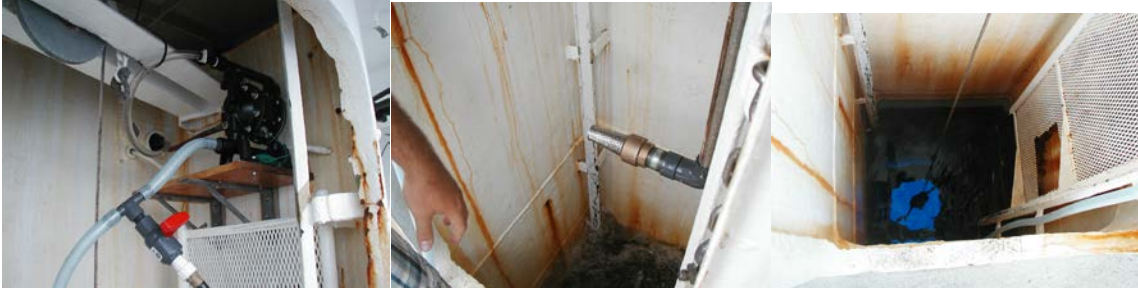
Figure 2. Moon pool aka Straza Tower (center and left), custom intake (center) and the compressed air driven diaphragm pump and hose installed for the flow through system on the Atlantic Explorer by Norm Nelson.
