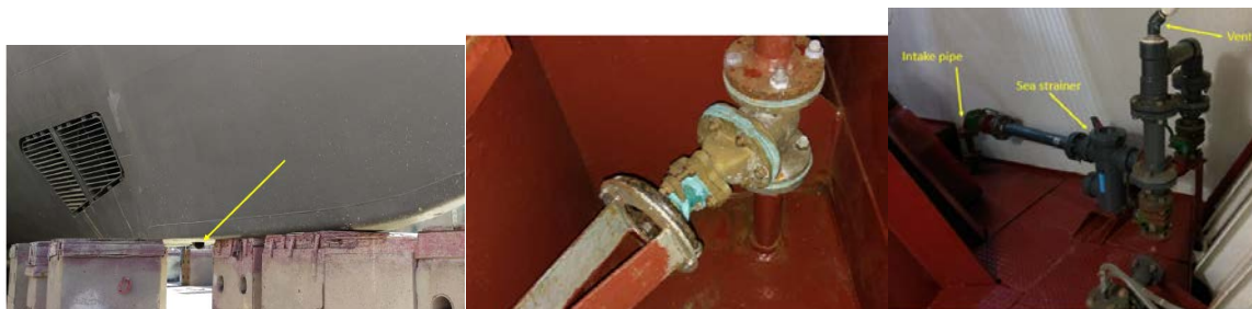
Figure 5. Intake scoop on the bottom of the vessel (left), intake pipe (center) and sea strainer debubbling and venting loop(right) of the R/V Atlantis.
